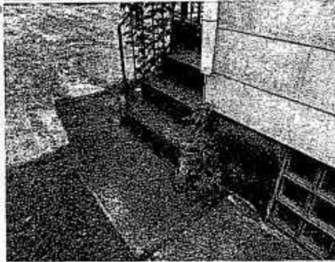
Iron carrier exhibits damage.
