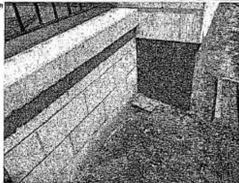
Foundation concrete exhibits damage, cracks, and/or is in danger.
