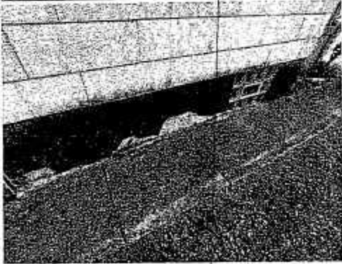
Masonry work exhibits damage.
