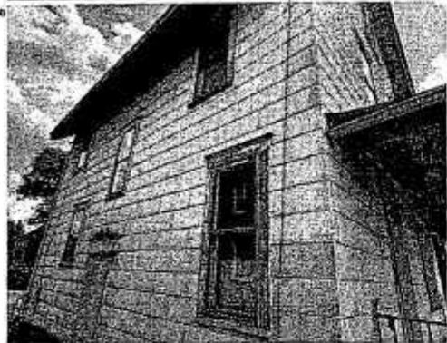
Frame structure is located so close, there is exposed wood surface.
