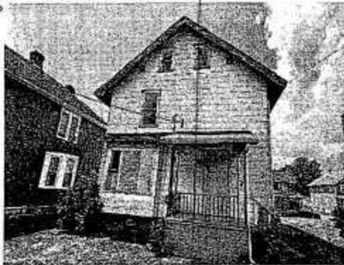
Major structure not bonded to code. Bare exposed wood surfaces.
